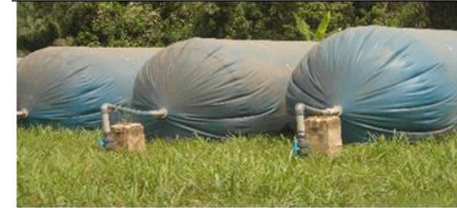
C: Biogas gasholders
