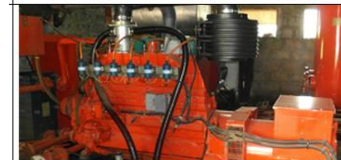
D: Gas generator
